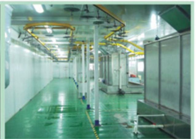
手動噴鍍懸掛綫 manual spray plating suspension line
