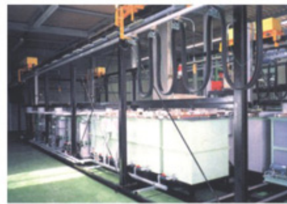
整廠電著塗裝自動線 Whole-plant electro-coating automatic line
